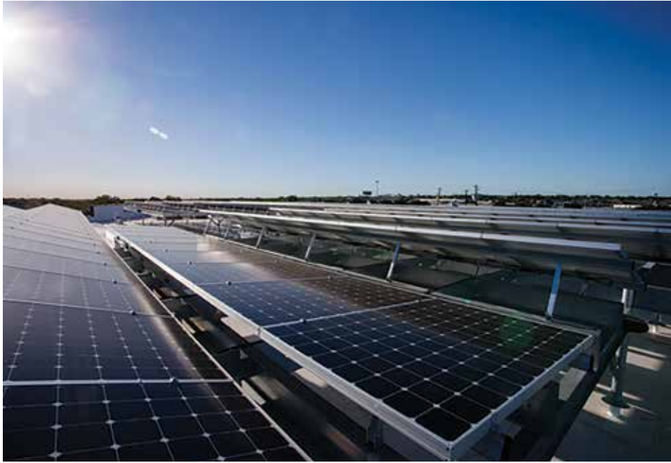
Padrón Elementary School Rooftop Solar Panels
