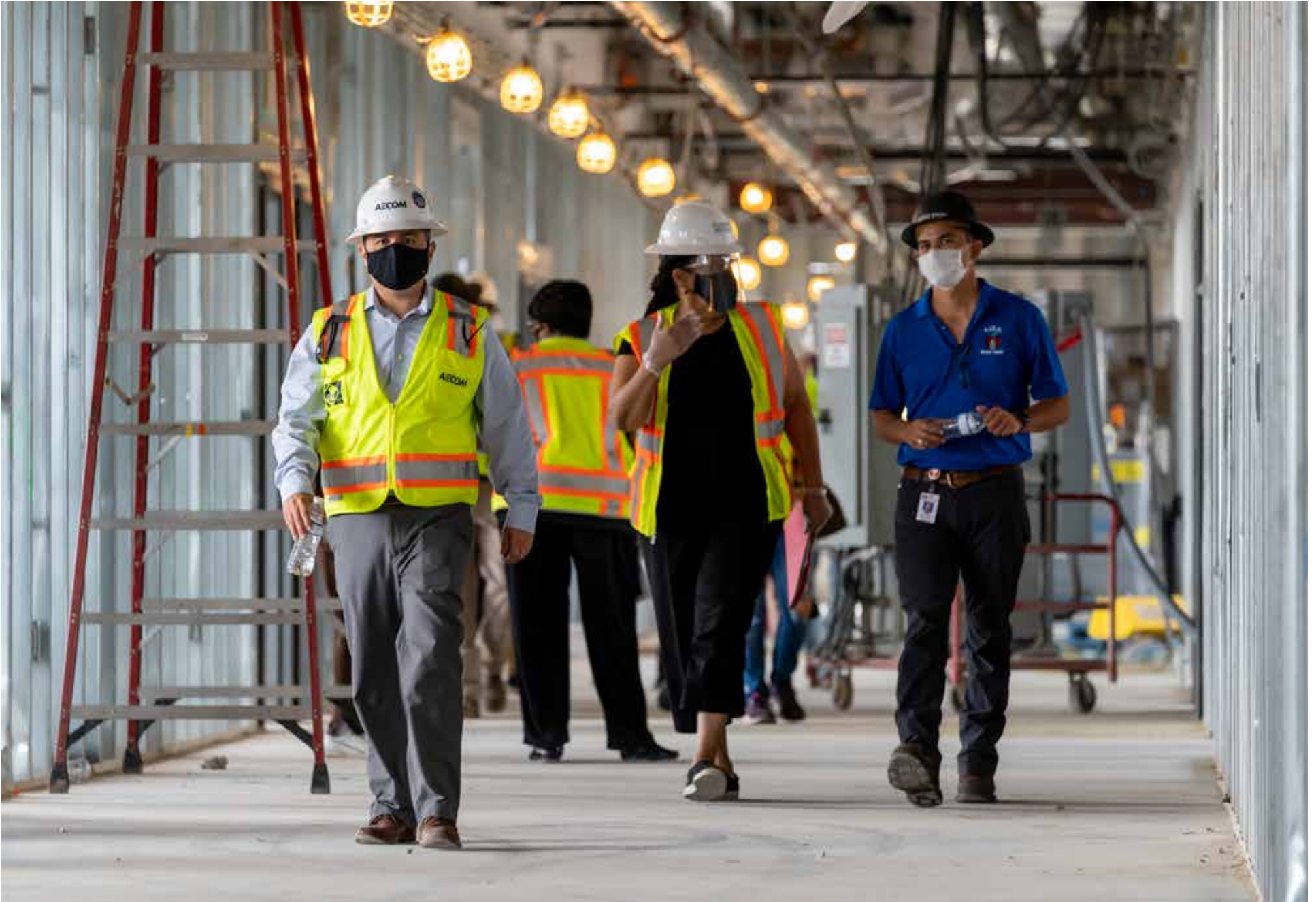
Eastside Early College High School at L.C. Anderson construction site tour: Carlos Mederes (AECOM), Barbara Spears-Corbett (L.C. Anderson Alumni), Matias Segura (AISD) tour the site.
