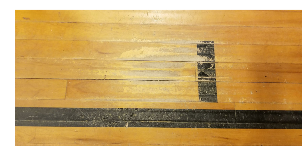
PHOTO 5: SAND FLOORING DOWN TO THE WOOD. REPAINT COURT MARKINGS TO "LIKE NEW" CONDITION.
