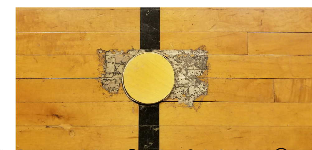
PHOTO 4: SAND FLOORING DOWN TO THE WOOD. REPAINT COURT MARKINGS TO "LIKE NEW" CONDITION.
