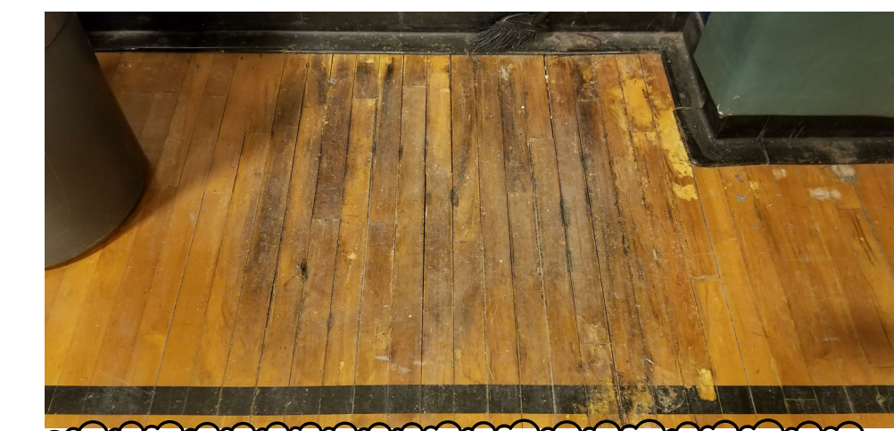
PHOTO 1: REPLACE DAMAGED FLOOR, MAJOR REPAIR / REPLACEMENT, RE: NOTE 6 OF GYMNASIUM FLOOR PLAN GENERAL NOTES.
