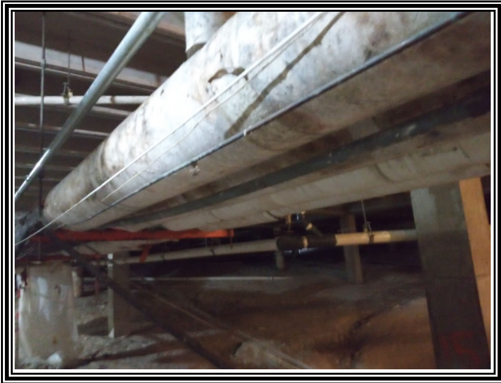
1. Pipe insulation inside the crawlspace was found to contain up to 2% chrysotile asbestos.
