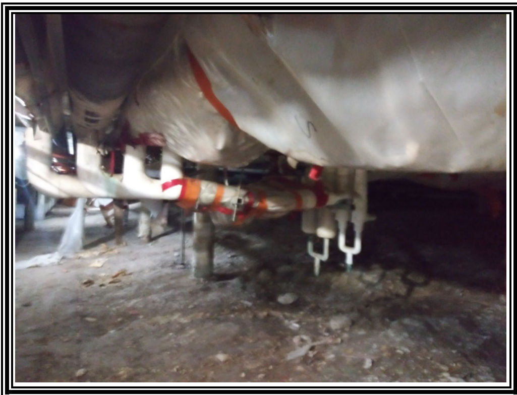
2. Pipe fitting insulation in the crawlspace was found to contain up to 2% chrysotile asbestos.
