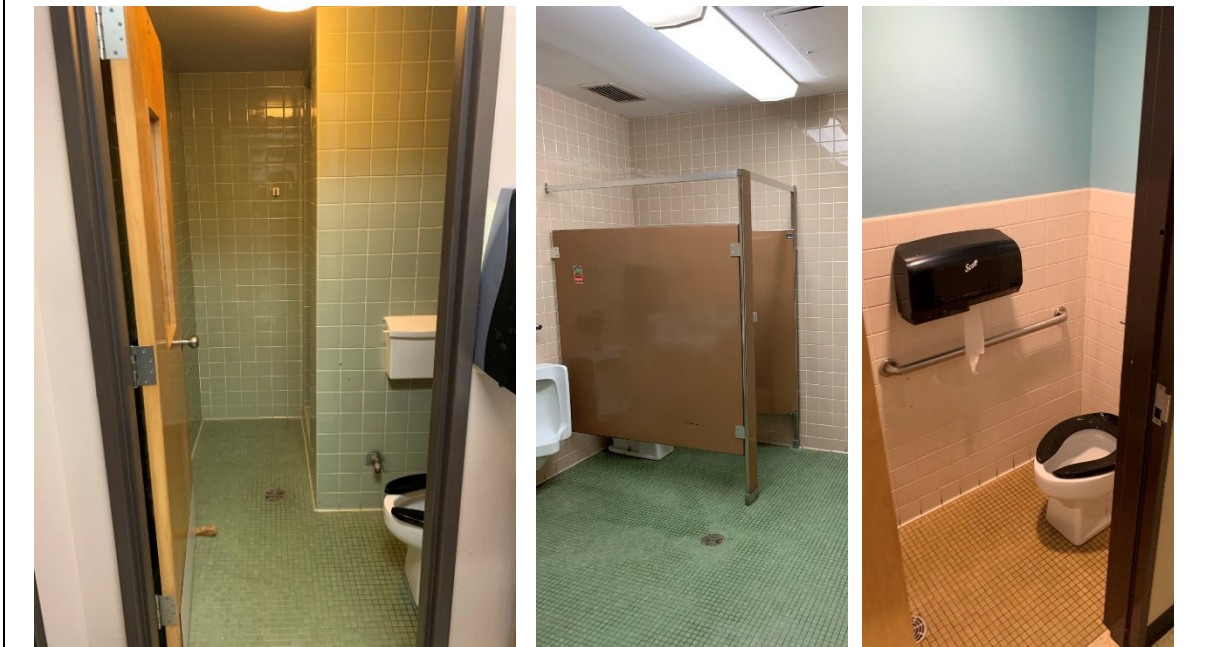
No restroom on campus appears to have adequate ADA accessibility. Accessibility will be covered within the Facility Condition Assessment but is noted here since it does not create an equitable use of space for all students.
