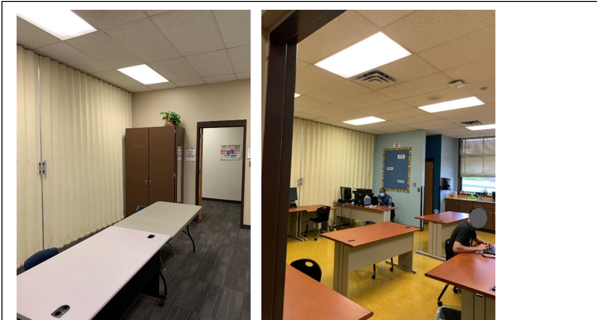
Typical studios with dated accordion partition. Typically kept closed due to sound transmission.
