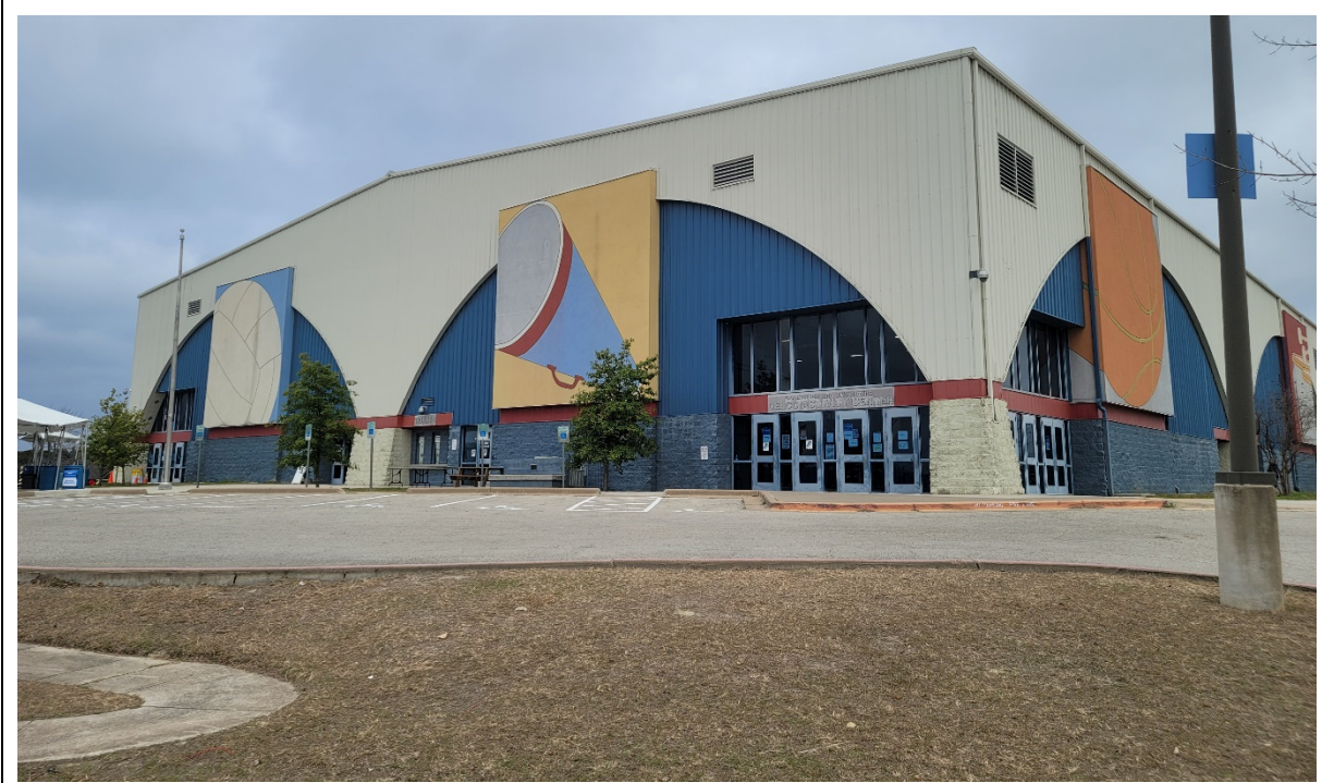
Overall exterior of the building is in good shape. Facility takes pride in the exterior graphics and the staff says they should be preserved.
