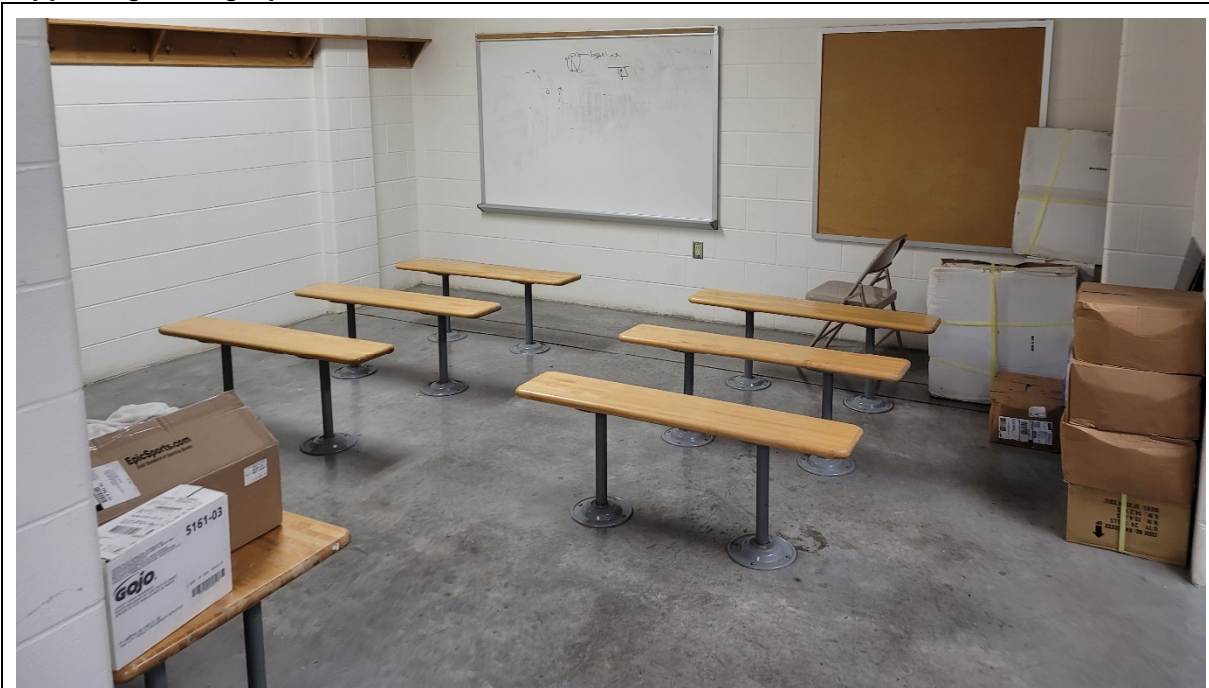
Locker room needs updates as well as additional storage.
