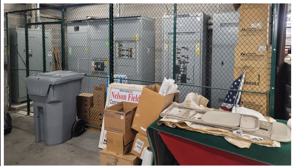
Storage area shares space with electrical panels and mechanical equipment. This makes it hard to do maintenance and stored items need to be moved.
