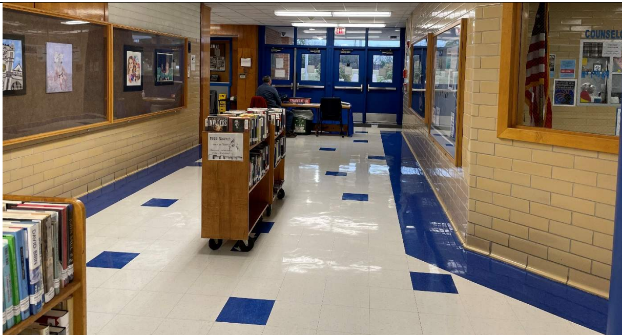
Main Entry is small and has a low ceiling and dated lighting.
