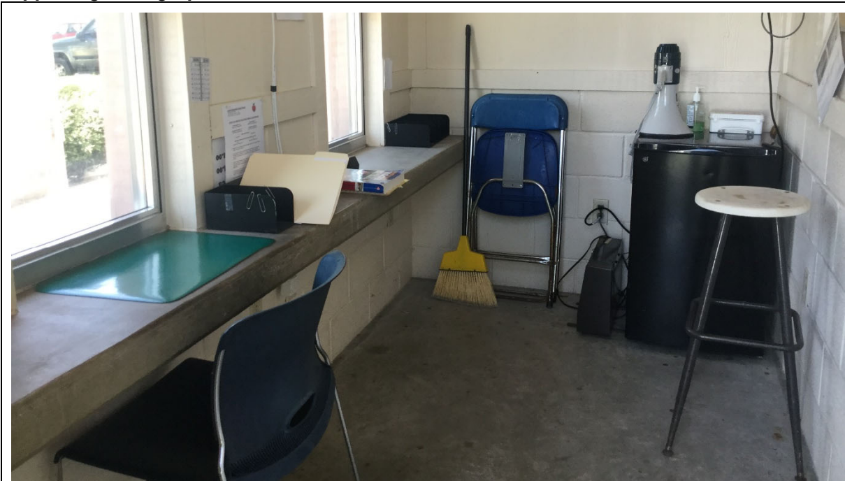
Ticket booth space is outdated and needs air conditioning.
