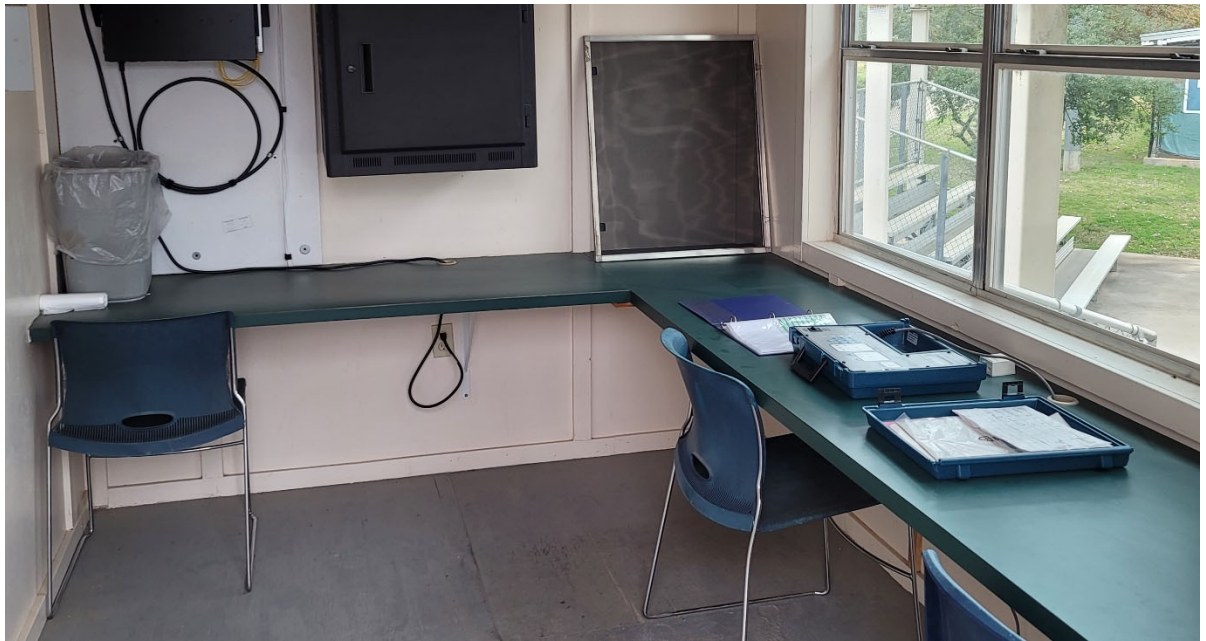
Softball press box needs to be conditioned. There is currently no AC or heat.
