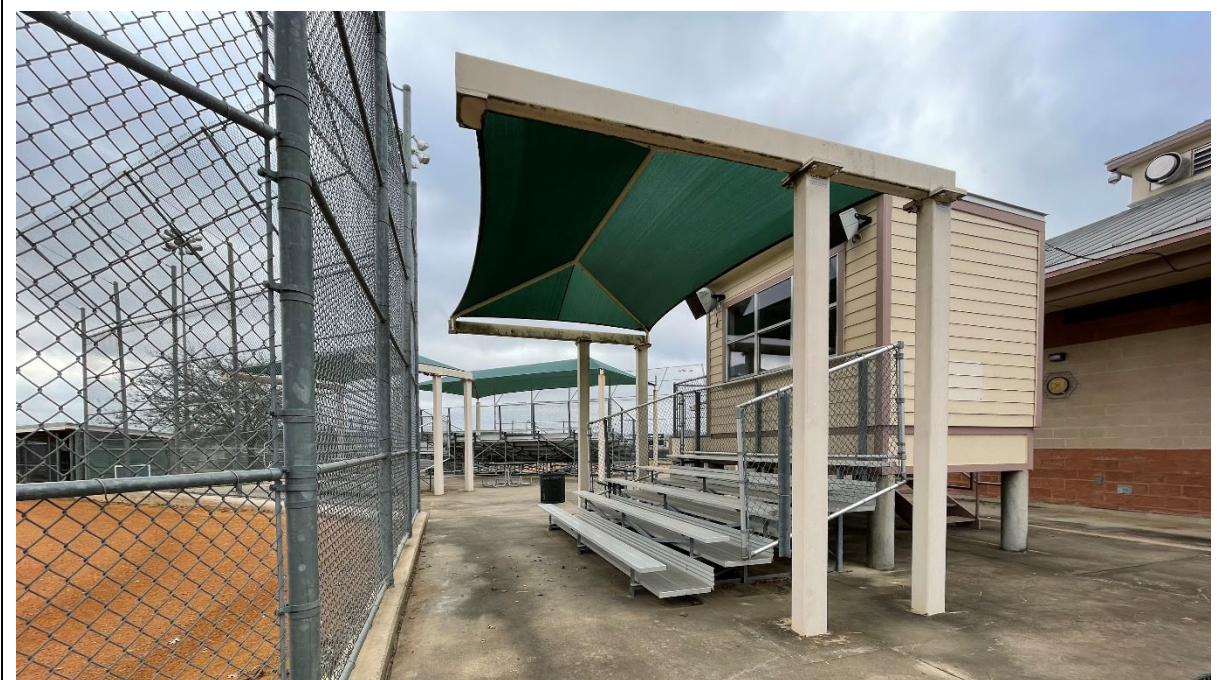
Softball bleachers are in good shape overall. There is rust and some wear on the shade and steel columns.
