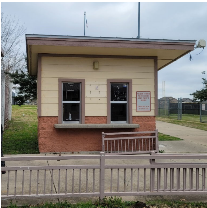
Exterior of ticket booth is in good condition overall; needs maintenance and [REDACTED]
