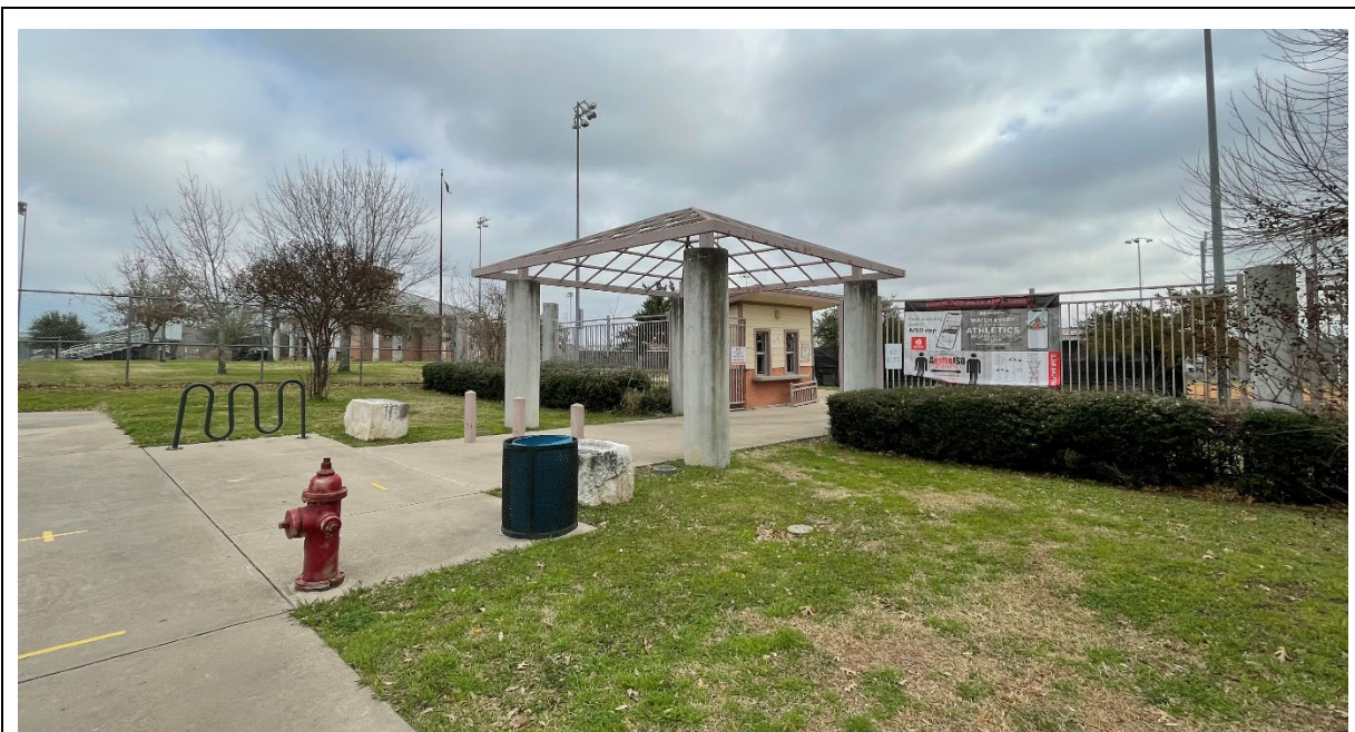
Entrance trellis columns are weathering and paint on steel is rusting and chipping.
