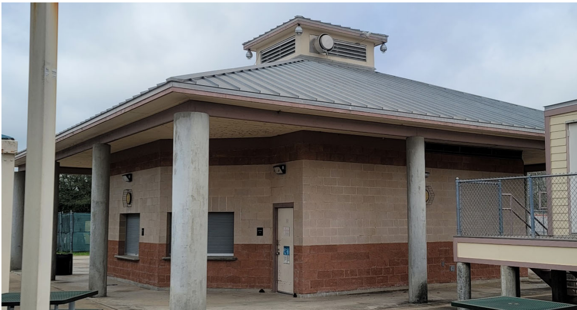
The building that houses concessions and restrooms shows wear and paint chipping on the outside.
