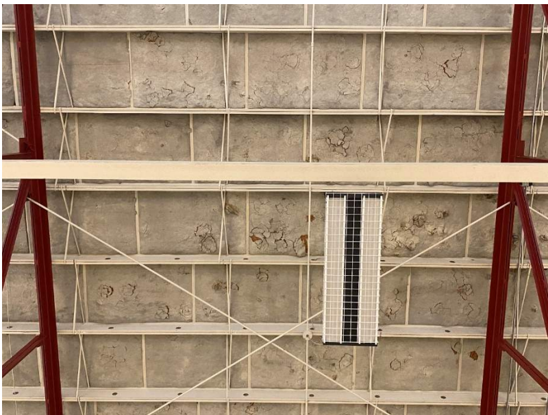
Aging building has noticeable maintenance and visual concerns, including aged insulation in gym ceiling. FCA will examine these issues more thoroughly, but they have negative visual impact and affect pride and learning environment.
