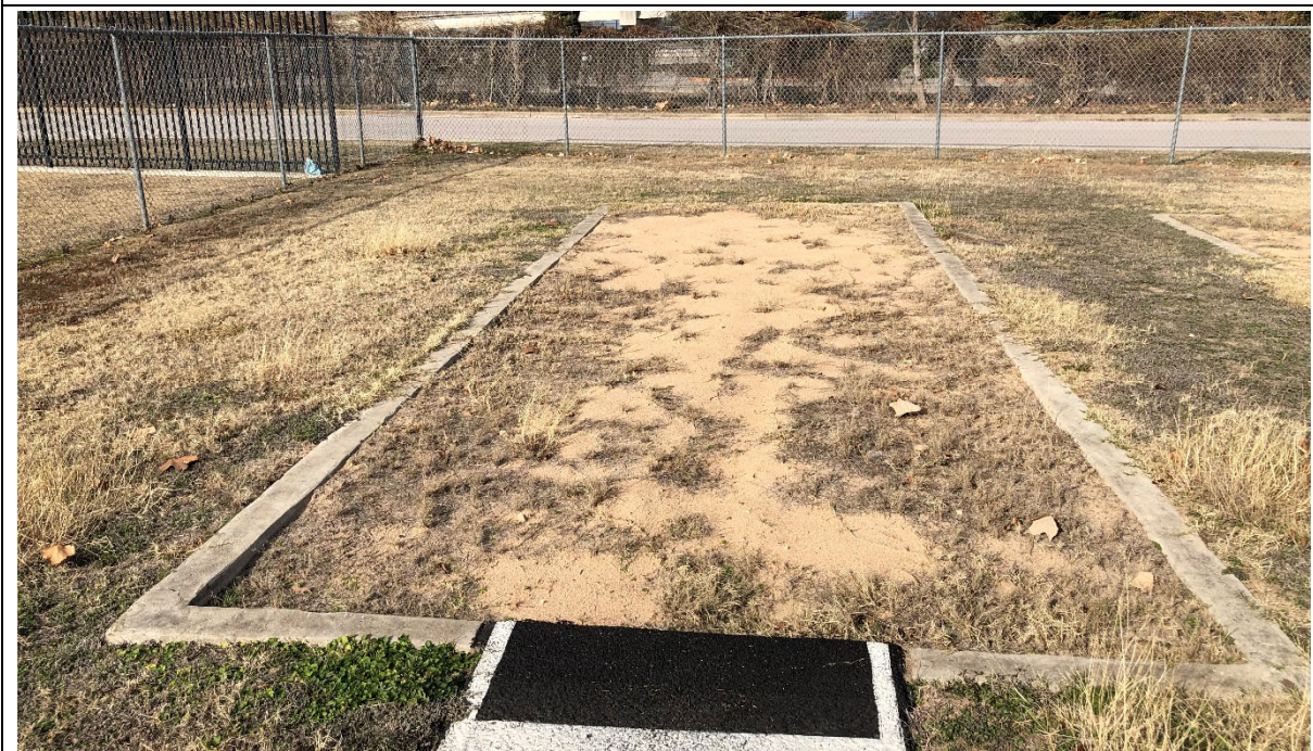
Landing at long jump runway needs maintenance with overgrowth of grass into sand pit.
