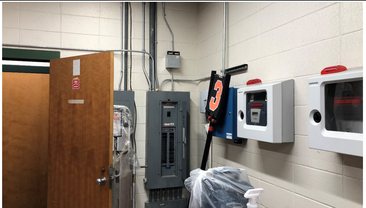
Electrical panels sharing space in the concession room.
