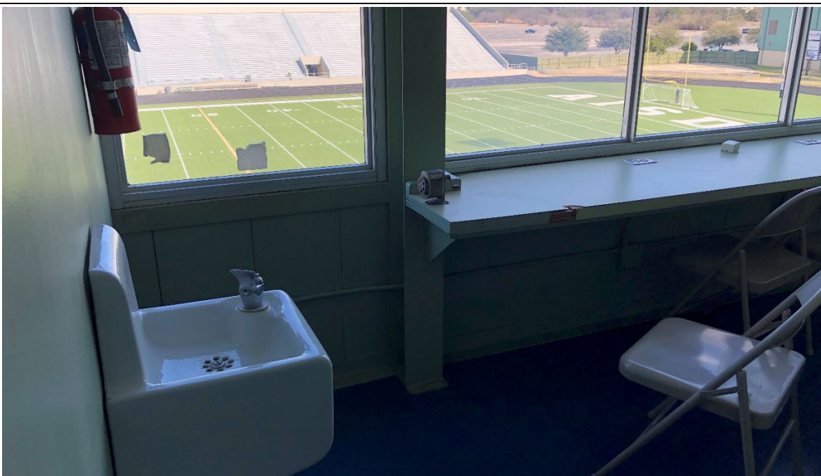
View of press box with dated fixtures and worn and deteriorating countertop.
