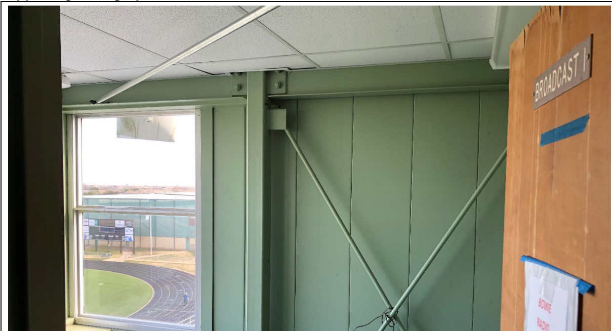
Broadcast space at press box with deteriorating door and exposed cables.
