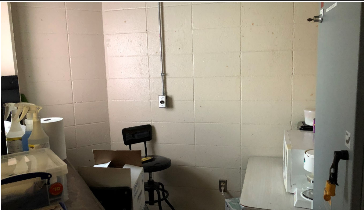
Electrical panel in ticket booth.
