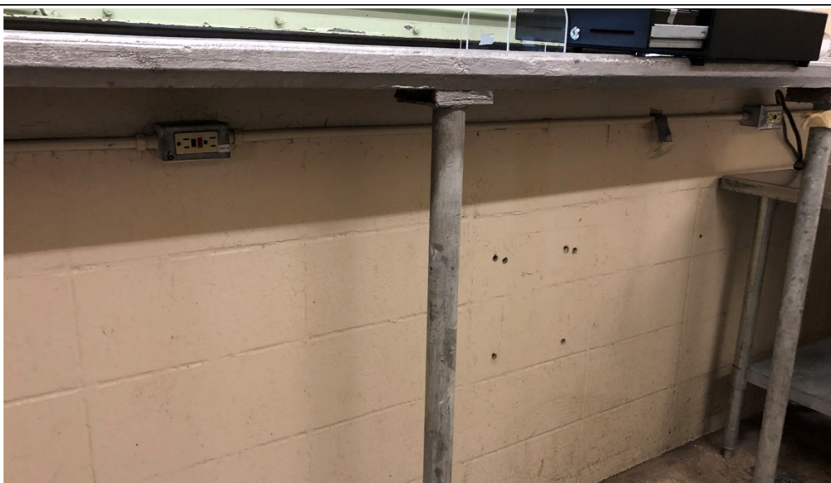
Power outlets not conveniently located under concrete counter at concession. Wall and posts stained and in need of painting.
