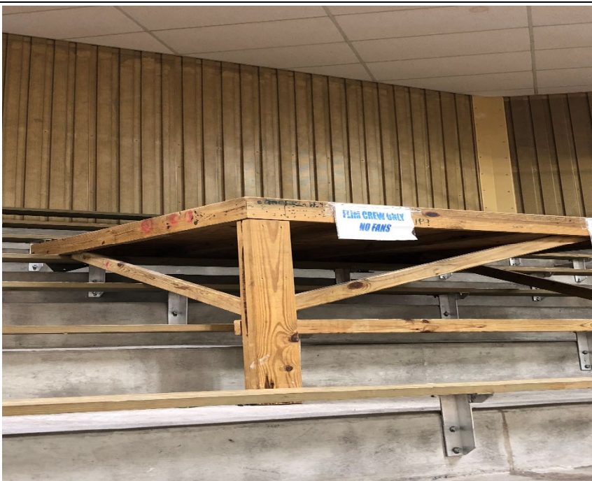
Film crew platforms in bleachers appear worn, unstable and not in good condition.
