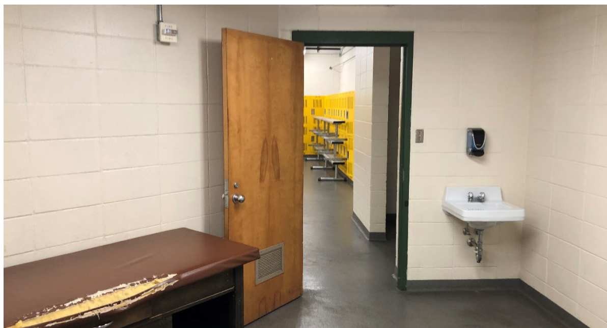
Other training room with torn equipment/furniture.
