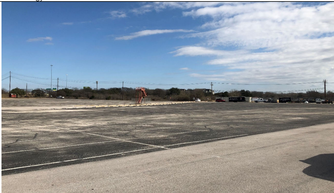
Condition of parking lot appears in fair condition. Some areas need repairs.
