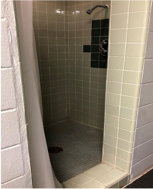
Officials' room shower with dated tile and in poor condition. Shower is not ADA-compliant.
