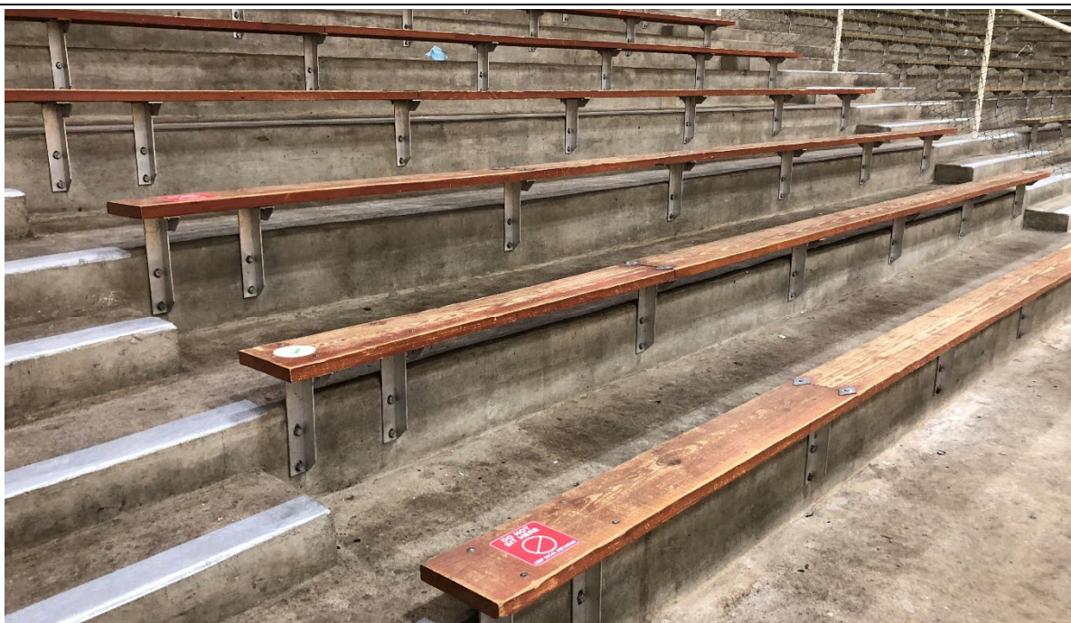
Seating in arena area old and in worn condition.
