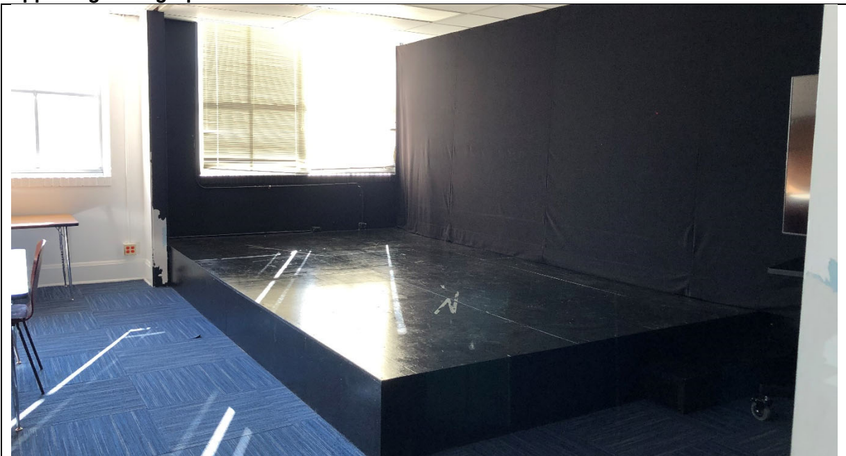
One of the studios is used as a flex space for performance practice. Makeshift stage was created with attempt to soundproof with carpet tile (not fully adhered) and fabric wall.
