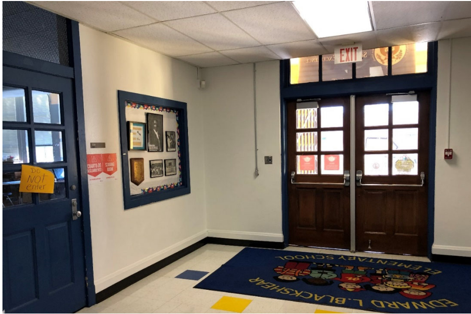
The main entry is small with a low ceiling and does not feel welcoming as an elementary school. The entry lacks a secure vestibule and is far from the main office. This layout allows visitors to enter without supervision.
