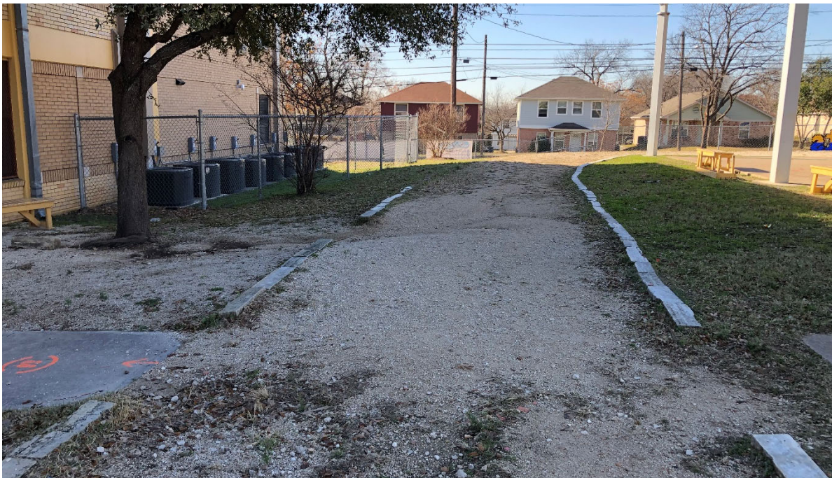
Track surface is eroding from rain runoff and is a hazard for users. The District Project Manager noted that this will be addressed in an upcoming improvement project.
