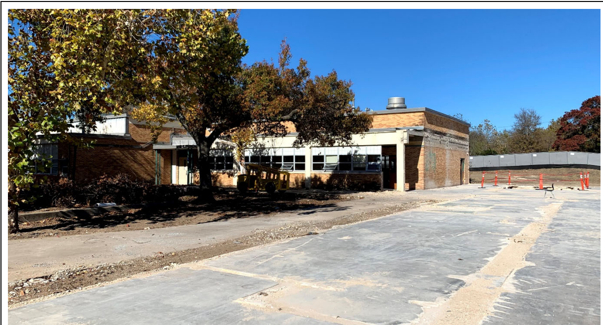
Exterior: East side of site – demolished structure. Addition to be located here.
