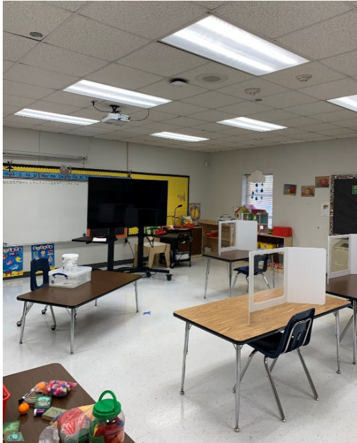
Furniture/Equipment: Dated or damaged furniture in main building. Some not correctly sized for grade level. Limits flexibility and is difficult to rearrange.
