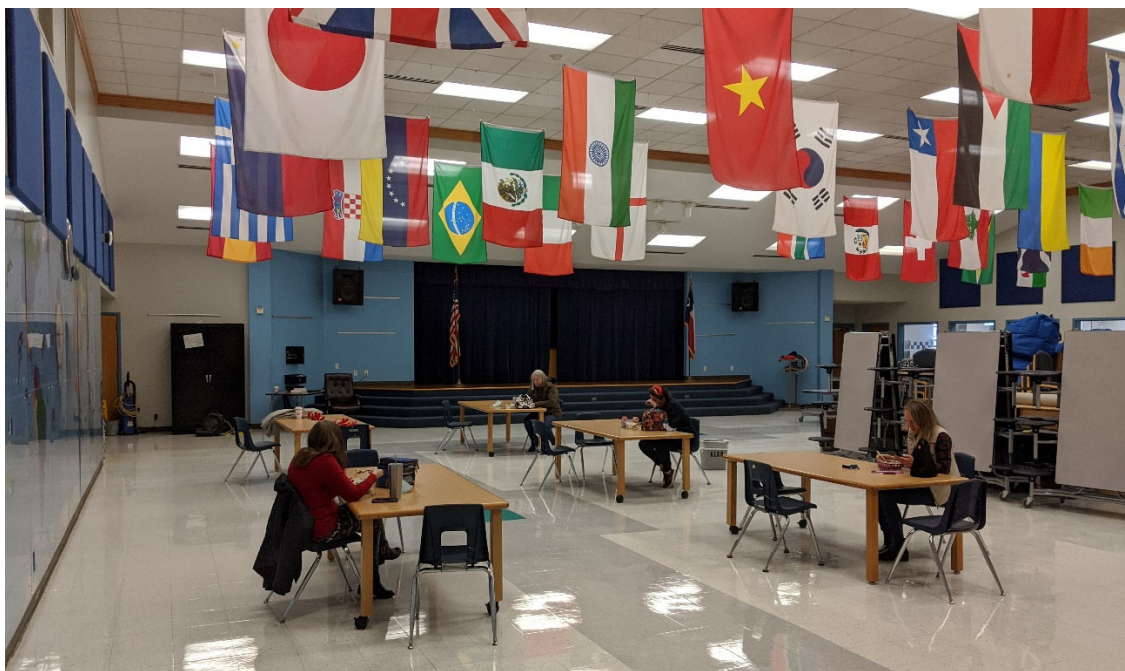
Food Services: Cafeteria is in good condition, but size does not meet Ed Spec based on current enrollment.
