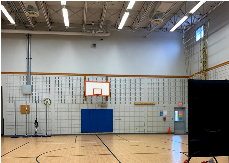
Gym is appropriately sized per Ed Spec but does not meet the current needs of the school. The gym and cafeteria open to one large space with an operable partition.
