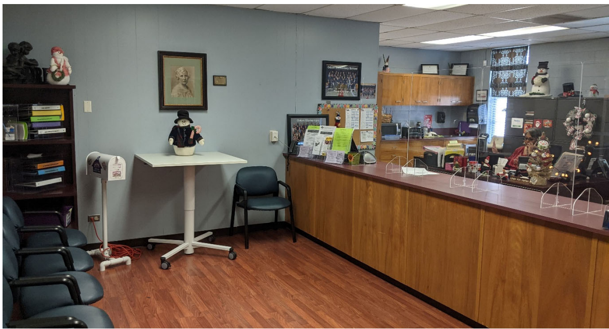
Administration Spaces: [REDACTED] The space has adequate seating, but furniture and finishes are dated.
