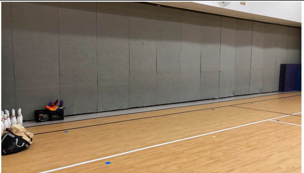
Operable partition between gym and cafeteria is deteriorating and not functioning properly. Difficult to open and campus typically keeps spaces separated.
