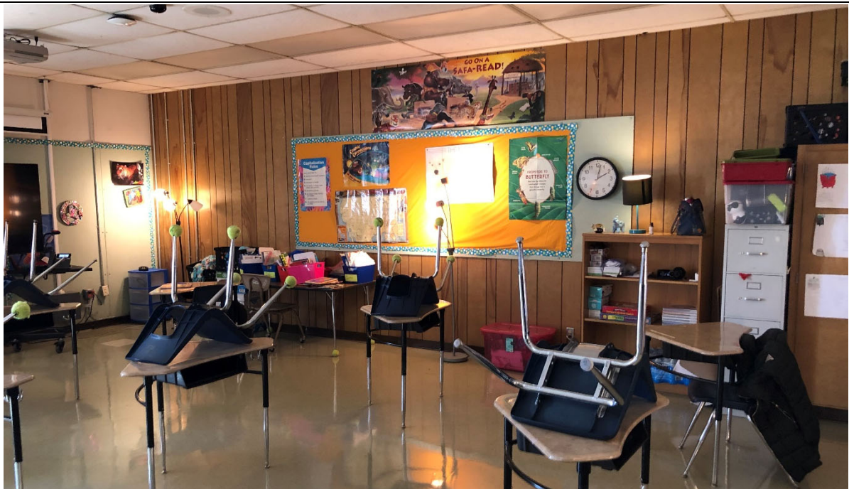
Studios in east wing have not been renovated to match west wing. Ceiling tiles, wall paneling and lighting are dated.
