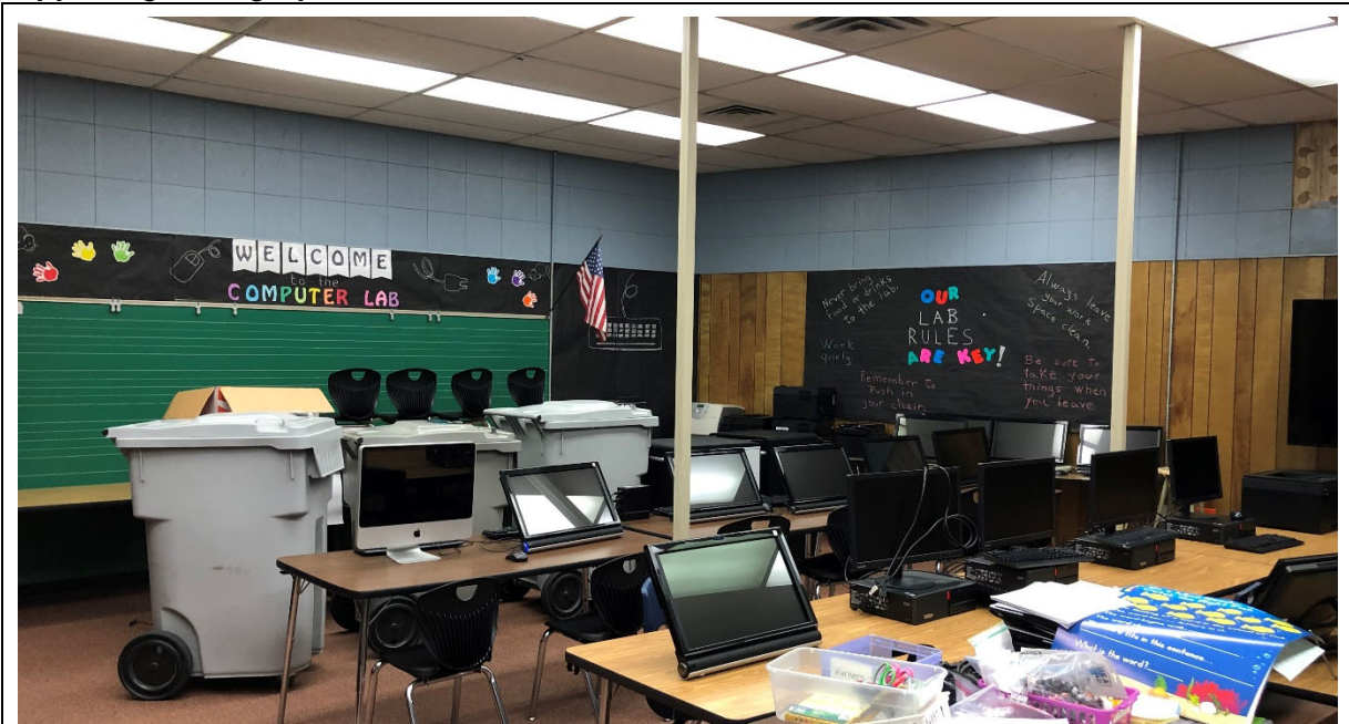
Computer lab finishes are dated. Thermal, acoustical and lighting quality are unsatisfactory and need attention. There was a strong odor in the room as well during the Assessment.
