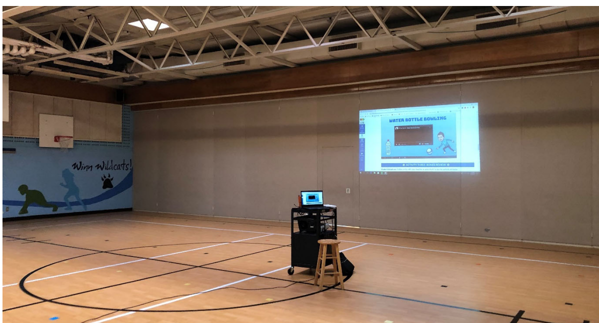
New floors in gym, but other surfaces need updating. It is undersized per Ed Spec at 2,200 SF. Acoustic control and ventilation are lacking.
