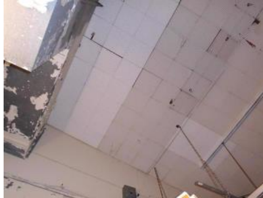
Ceiling accoustical tiles aged
