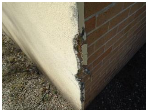
Broken and aged exterior wall
