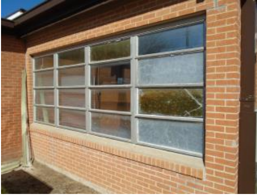
Broken exterior aluminum windows
