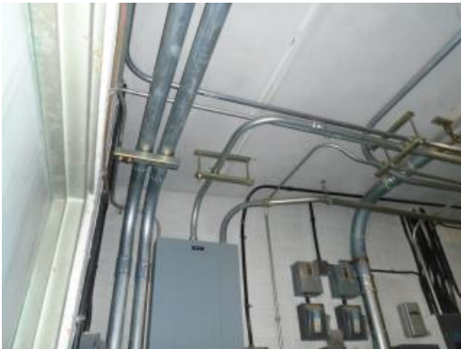
Aged electrical system
