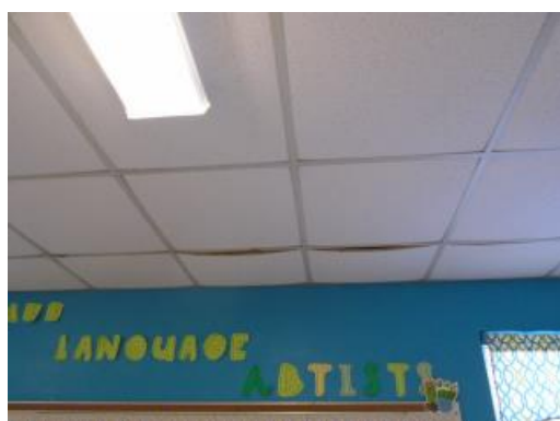
Sagging classroom ceiling tiles
