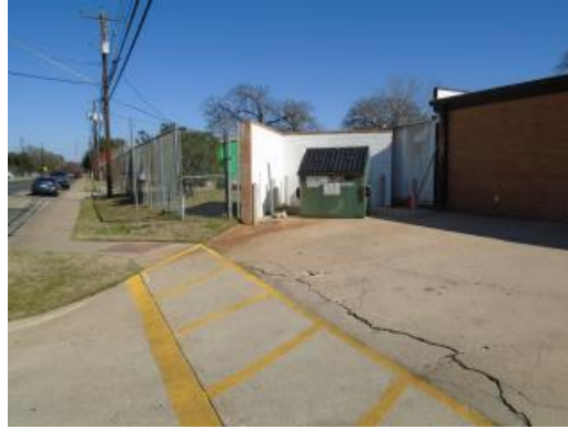
Cracked concrete driveway
