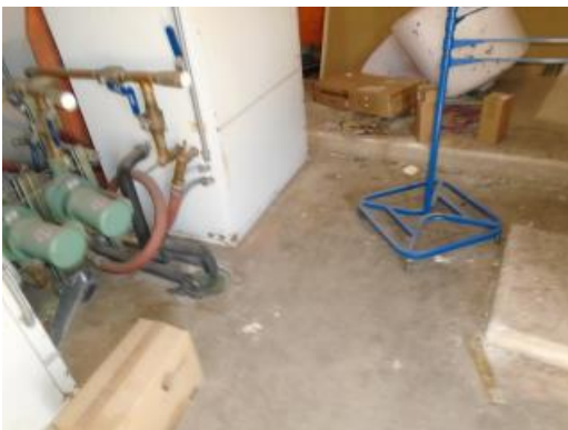
Old domestic water pumps at end of life
