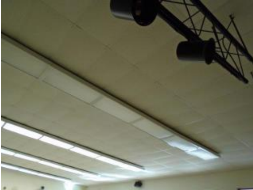
Ceiling lights out
