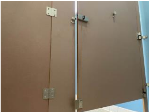
Restroom partition wall at end of life
