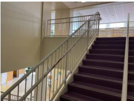
Stairwell railing missing paint and is aged
