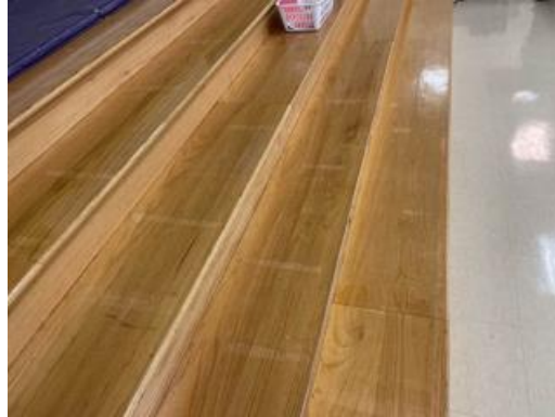
Deficient wood stage
