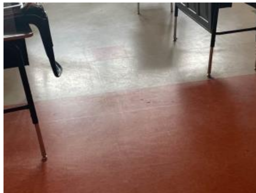
Vinyl composition tile flooring at end of life
