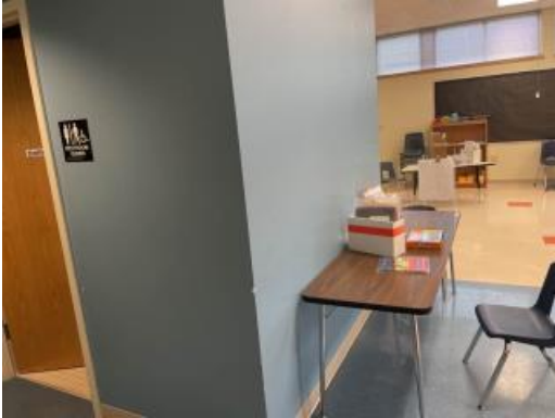
Nicks and peeling paint in classrooms
