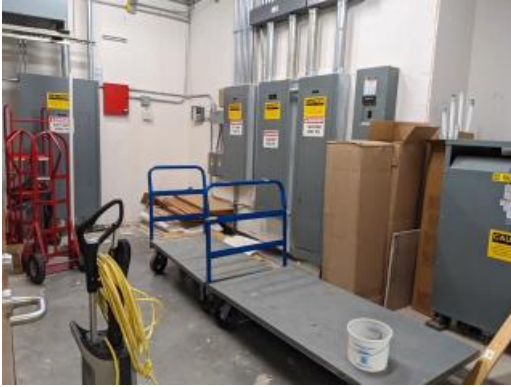
Obstructed electrical panels
