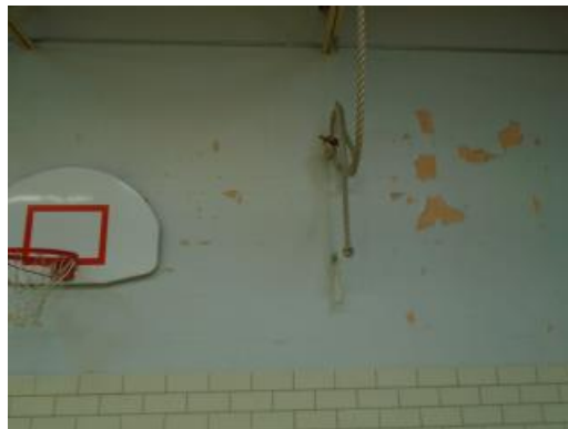
Peeling wall paint
