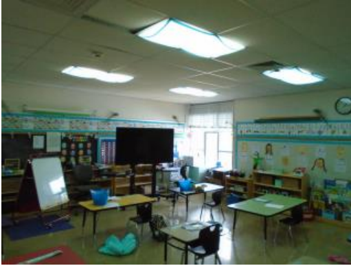
Broken classroom interior lighting and ceiling tiles
