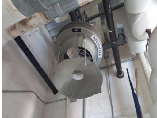
Corroded unit heater pipe
