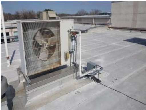
Libert unit corroding
