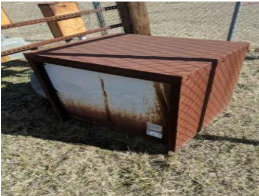
Outdated exterior transformer
