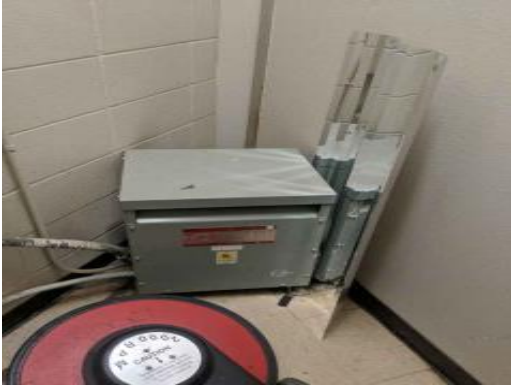
Electrical room equipment
