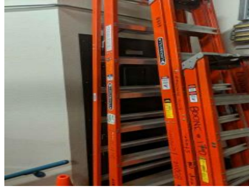
Obstructed electrical panel at stage
