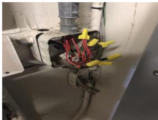
Unsafe uncovered wires
