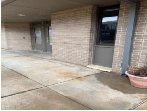
Evidence of water staining on concrete
