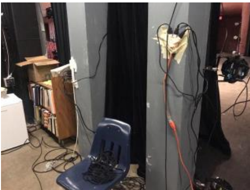
Unsafe wire pathways
