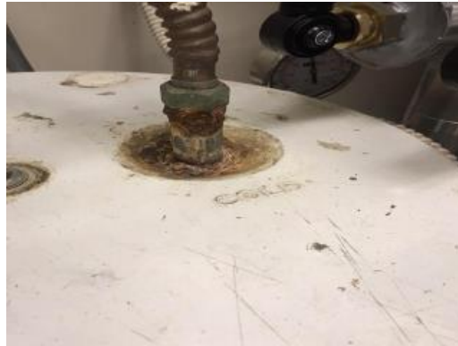
Corrosion on water heater
