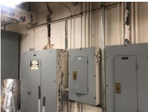
Electric panels approaching end of useful life
