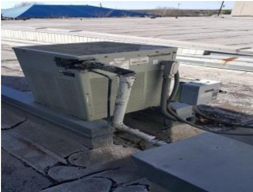
Condensing Unit R-22
