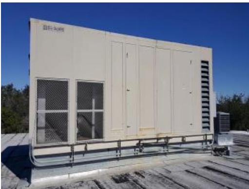
Dedicated Outdoor Air System
