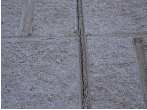
Damaged exterior wall caulking
