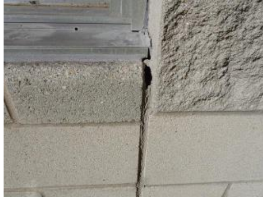
Damaged Exterior wall caulking
