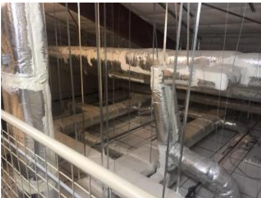
Above Ceiling ductwork
