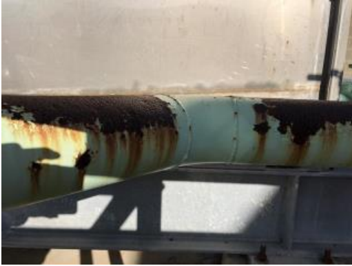
Rusted exterior pipe
