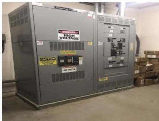
Main Switch Gear
