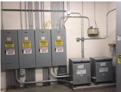
Electrical Panels and Transformers
