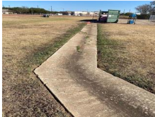
Stained concrete walkway
