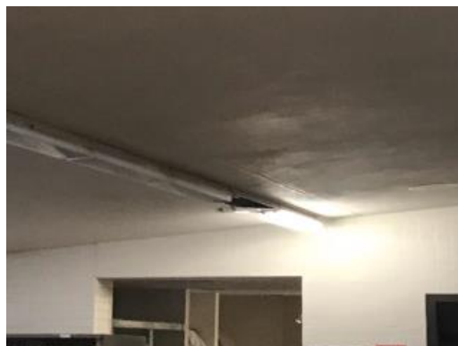
Warped plaster ceiling
