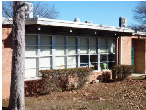
Aged Exterior windows
