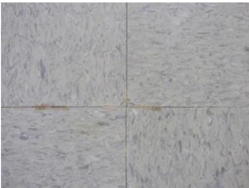
Damaged vinyl composition tile flooring
