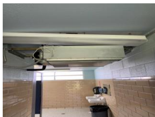
Mechanical equipment beyond useful life
