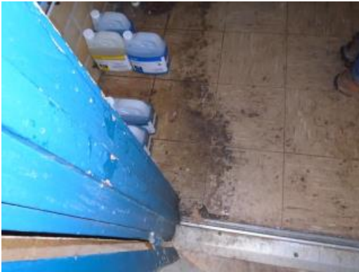
Damaged wooden door frame and floor tiles
