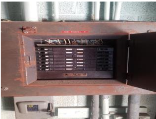
Aged electrical panels
