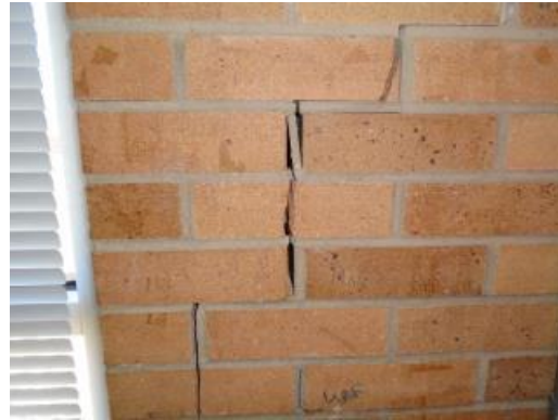
Mortar failure on brick
