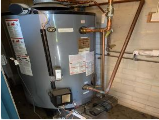
Aged water heater
