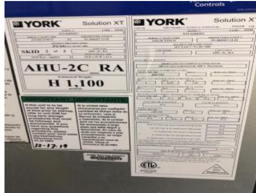
Air handling unit name plate
