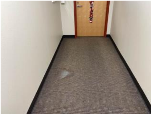
Carpet stain due to water leak above
