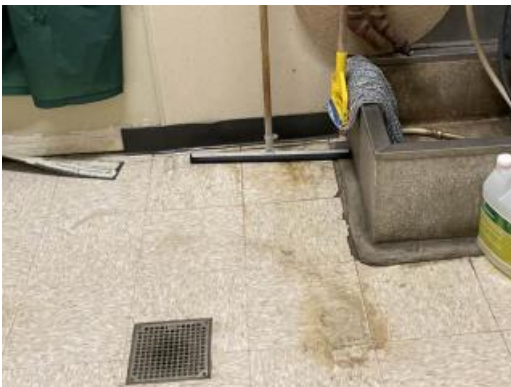
Vinyl composition tile flooring is stained
