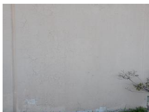
Paint on exterior walls is chipped
