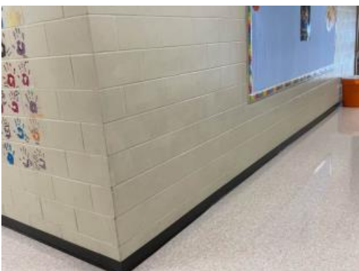
Third floor 800 hall wall is faded and should be repainted.
