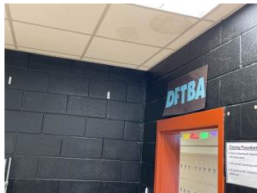
Acoustic ceiling tiles are stained
