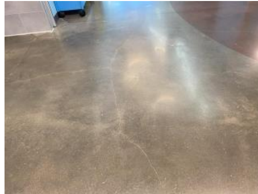
Concrete floor is beginning to crack.
