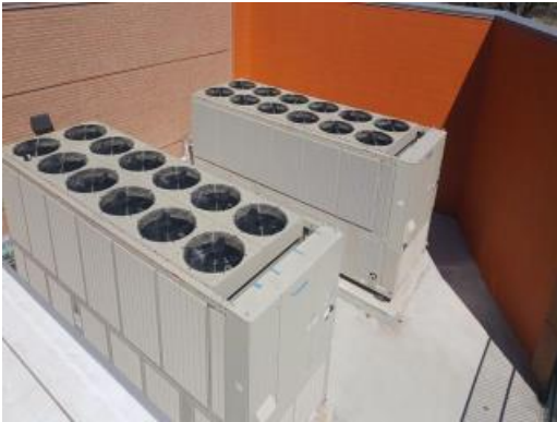
Air Cooled Chiller
