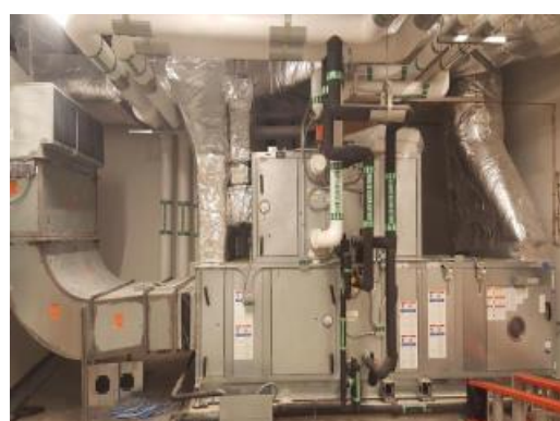
Indoor Air Handling Unit
