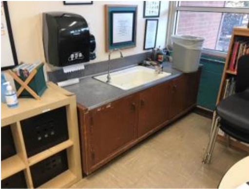
Classroom cabinets are beyond service life.
