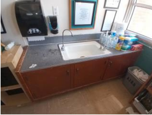
Sink and casework
