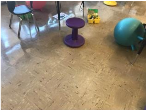
Classroom vinyl asbestos tile flooring is beyond service life.
