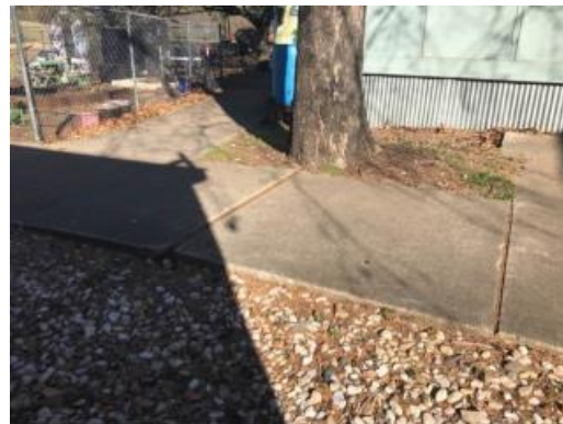
Site sidewalk is damaged and is a trip hazard.
