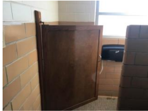
Class restroom partitions are beyond service life.
