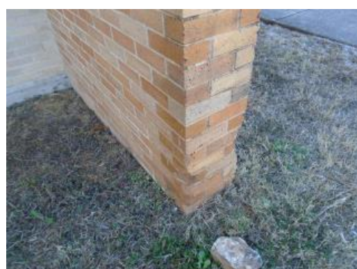
Worn and damaged exterior brick
