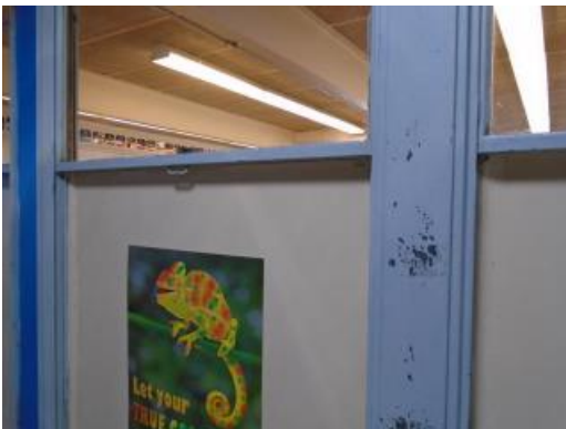
Worn paint on walls
