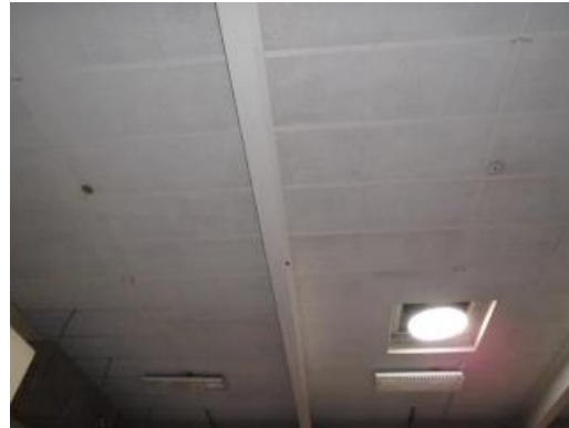
Slight discoloration on hard ceiling tiles
