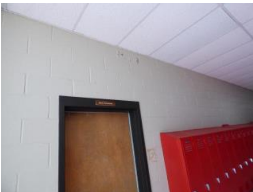
Concrete masonry unit (CMU) wall with slight damage
