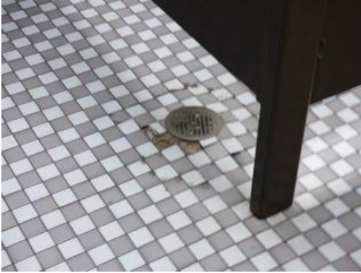
Ceramic tile (CT) is missing and cracked
