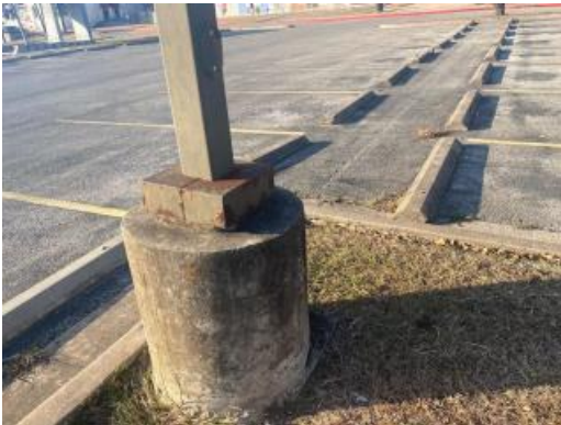
Light pole base is stained
