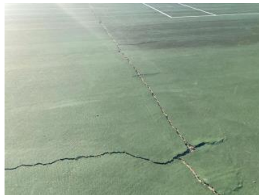
Tennis court surfacing is cracked
