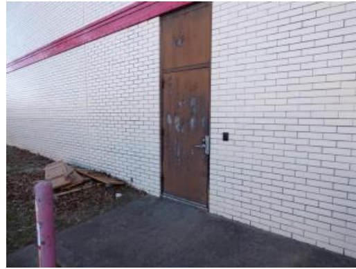
Exterior doors are worn
