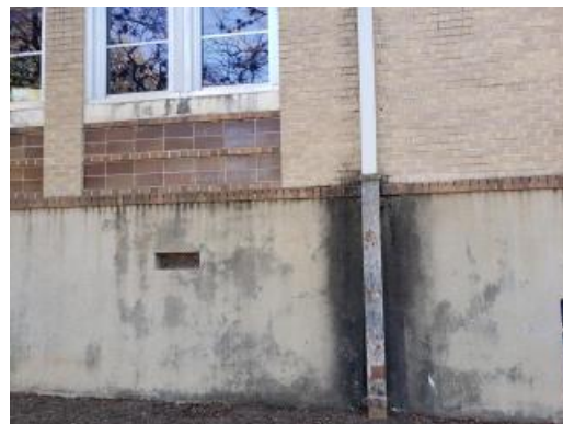
Stained exterior walls
