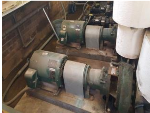
Circulating pumps at end of their life
