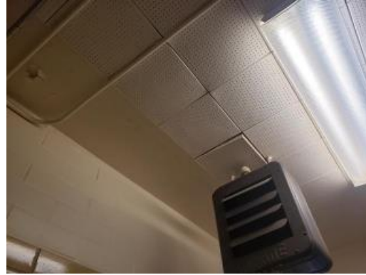
Aged acoustic ceiling tiles
