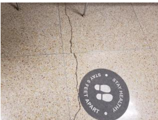
Cracked floor tiles
