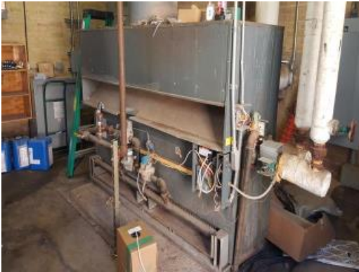
Boiler at end of its life
