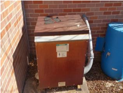
Electrical transformer aged
