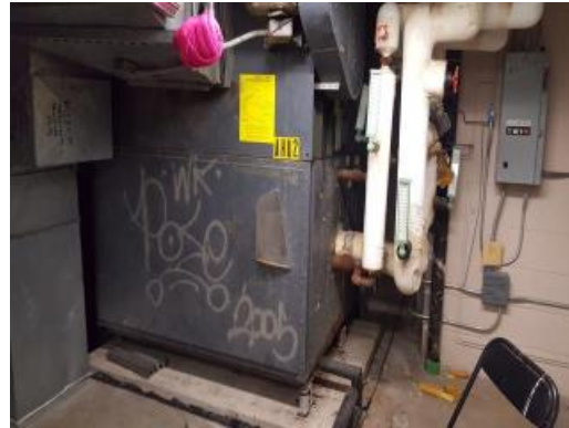
Air handling unit beyond useful life
