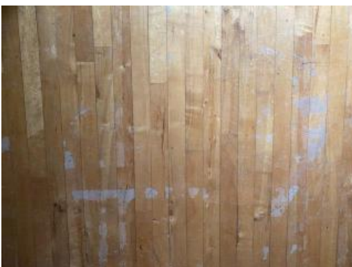
Wood floor worn and stained
