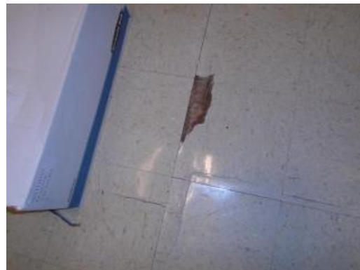
Damaged vinyl composition tile flooring
