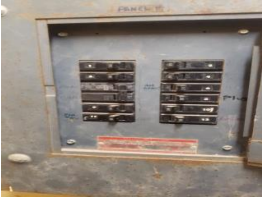
Aged distribution panel
