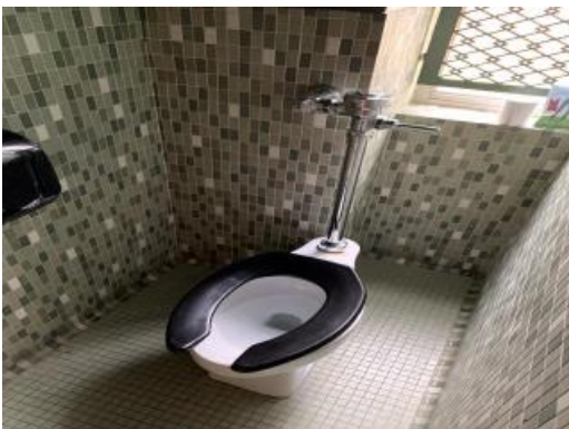
Aged plumbing fixtures
