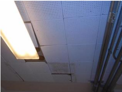
Glued ceiling tiles are damaged and missing
