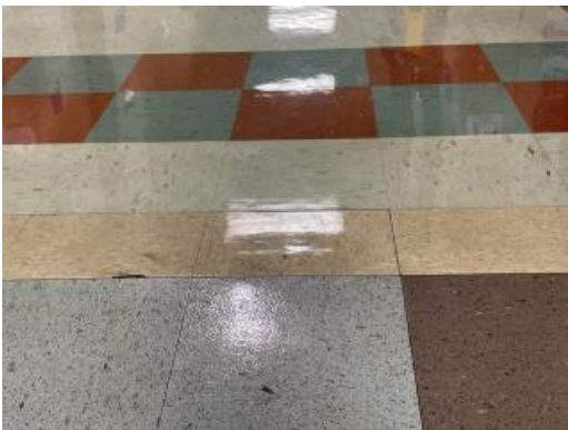
Worn vinyl composite tile is chipped
