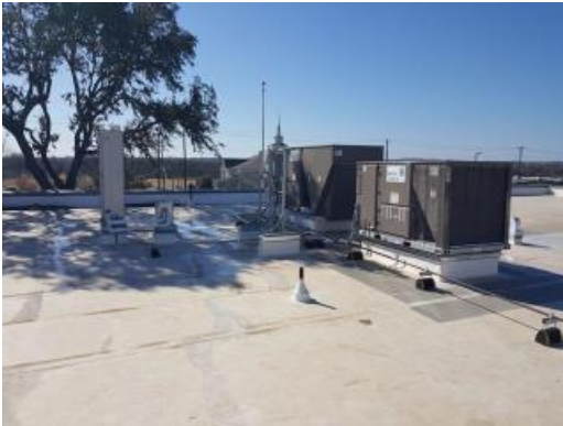
Rooftop heating ventilation and air conditioning units
