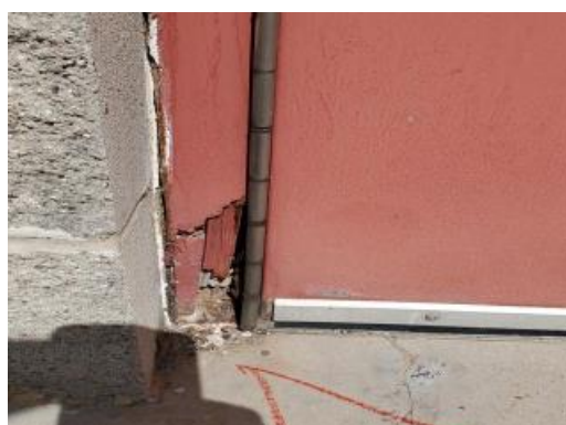
Damaged exterior door frame
