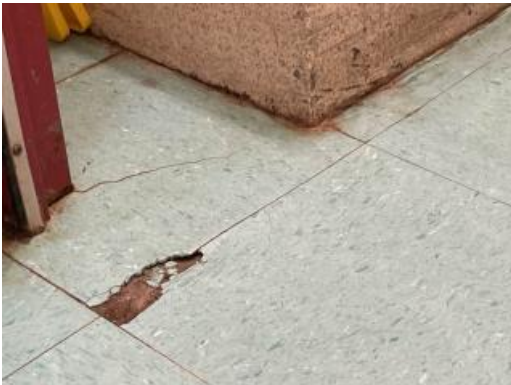
Damaged vinyl composite tile
