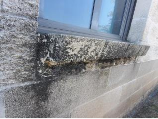
Stained exterior concrete wall
