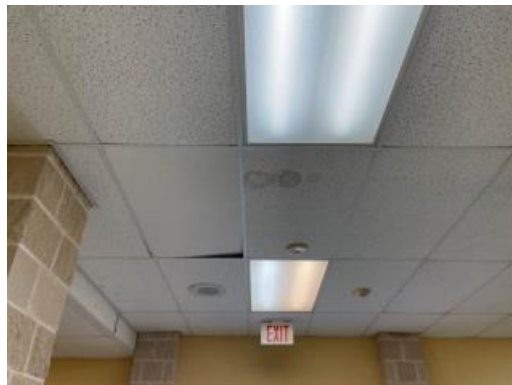
Damaged acoustic ceiling tile
