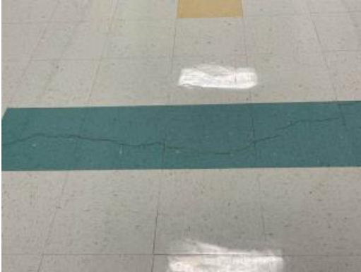
Cracked vinyl composite tile
