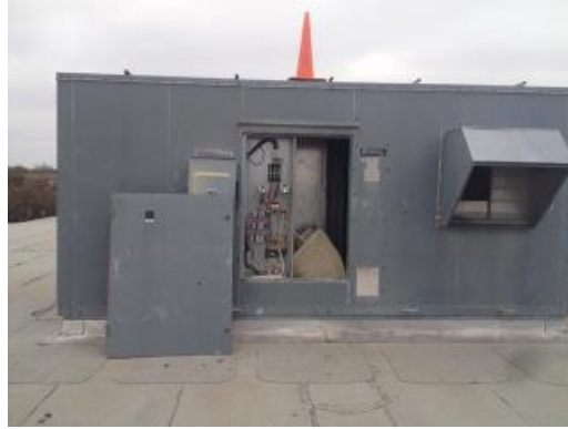
Exposed electric box on roof
