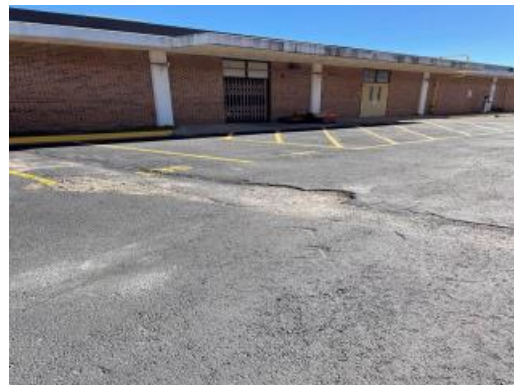
Aged asphalt paving
