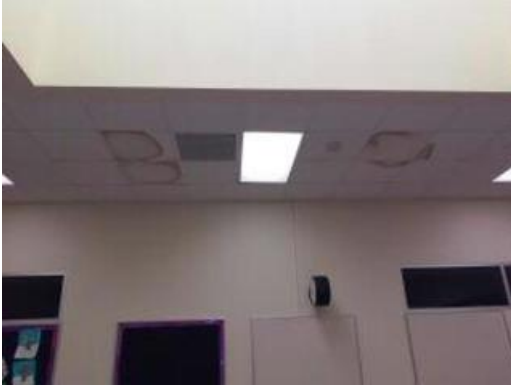
Stained acoustical tile flooring
