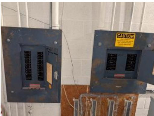
Aged electrical distribution panels
