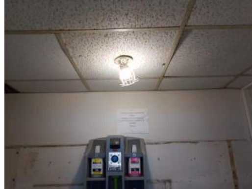
Aged acoustic ceiling tile
