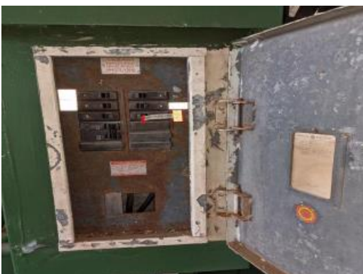
Electrical panel is past useful life
