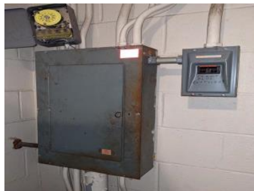
Electrical panel is rusted
