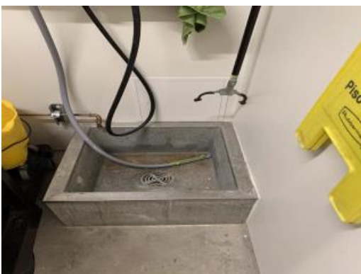
Mop sink is worn
