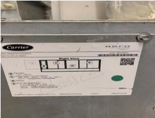
Air handling unit name plate
