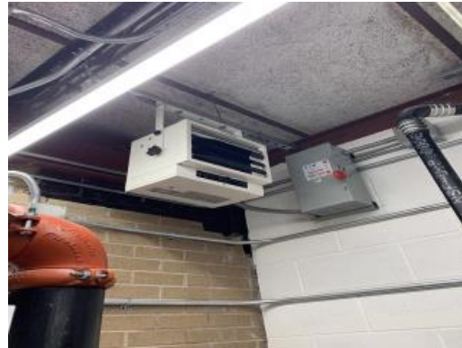
Unit heater is aged
