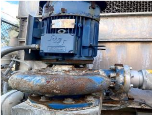
Pump is beyond its service life
