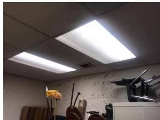
Peeling wall paint
