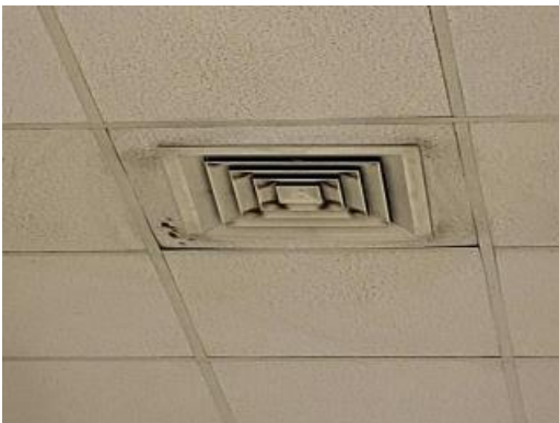
Water Damage to acoustical ceiling tile containing vent
