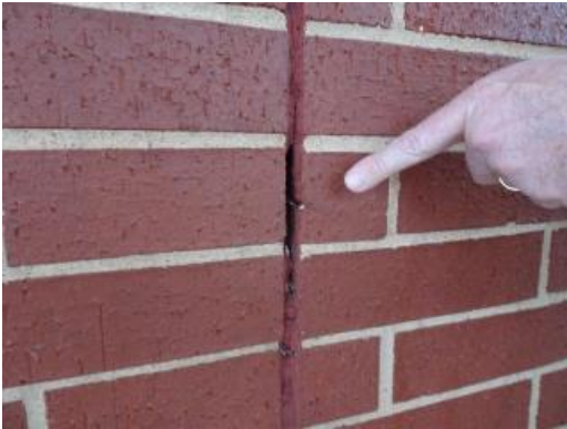
Damaged control joint
