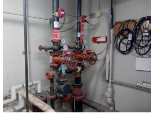
Fire riser system
