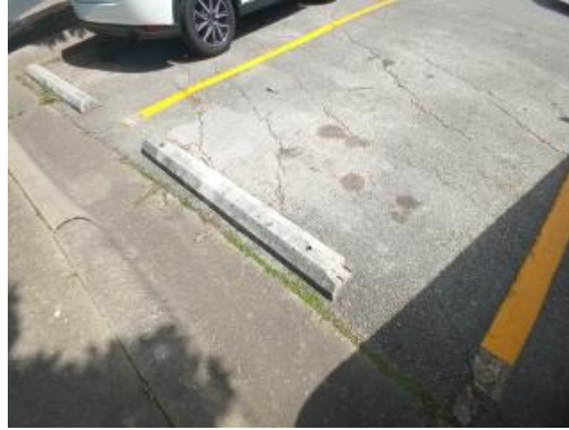
Pavement damage present
