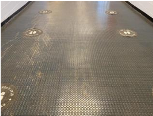
Worn rubber flooring
