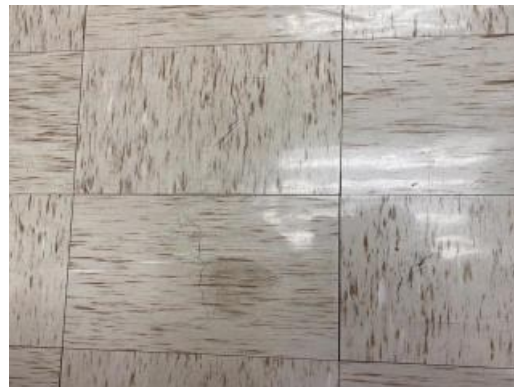
Damaged vinyl composite tiles
