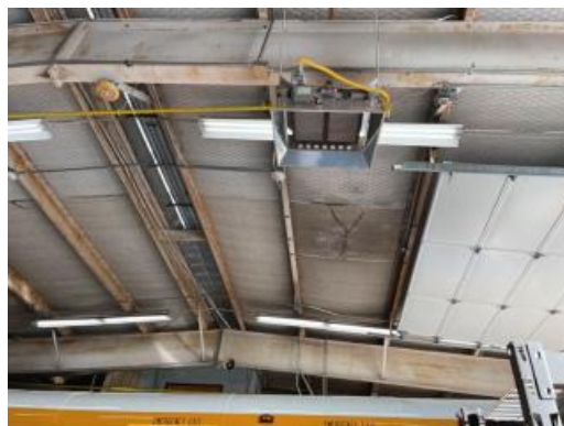
Shop ceiling insulation panels damaged
