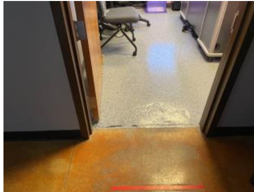
Damaged epoxy floor
