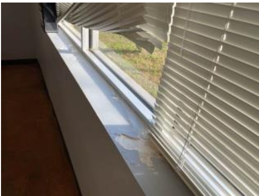
Damaged interior window seals due to water leak
