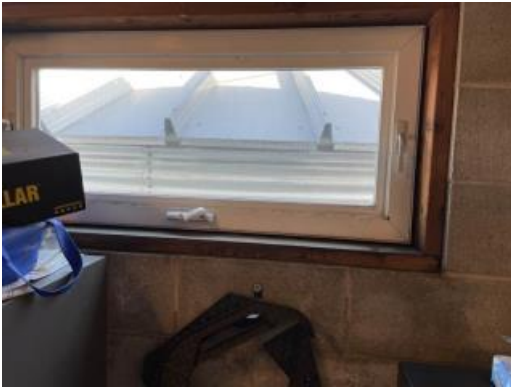
Mildew on window seal
