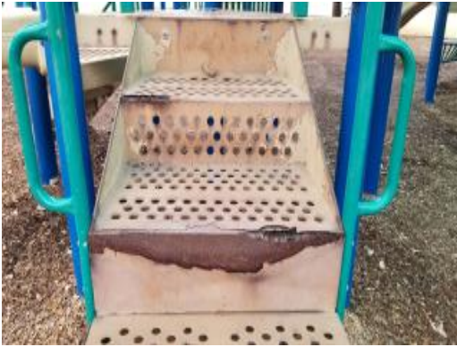
Playground rusted steps
