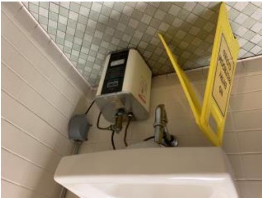
Exposed use water heater.
