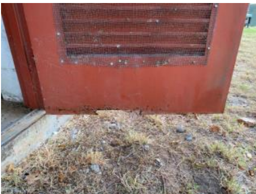
Corroded exterior door.
