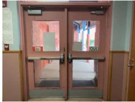
Exterior metal doors in need of re-finishing.
