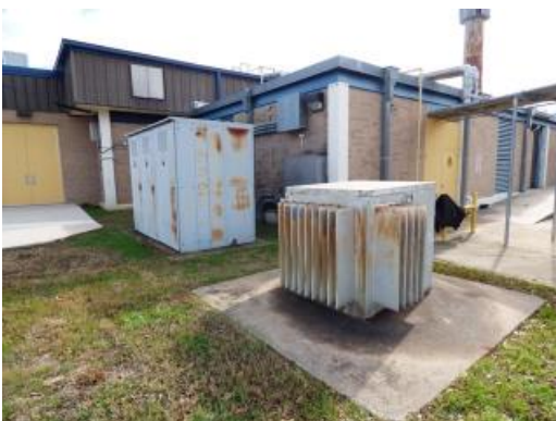
Aged exterior electrical service
