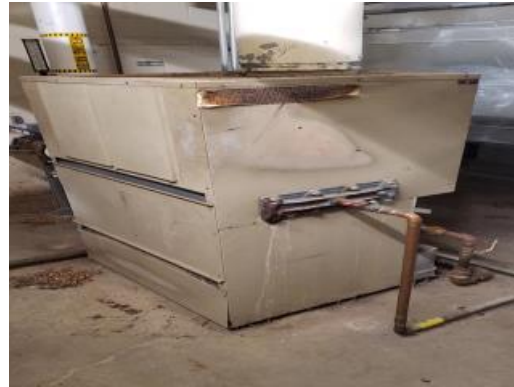
625 MBH boiler at end of life
