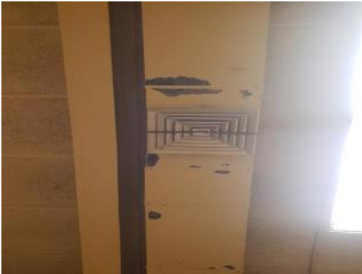
Ductwork is at end of life
