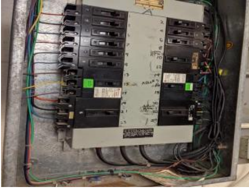
Exposed electrical panel
