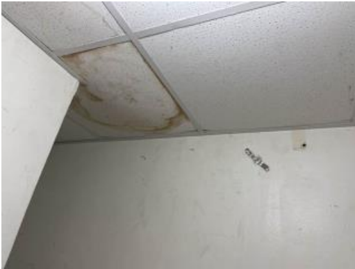
Stained main office admin mechanical closet ceiling
