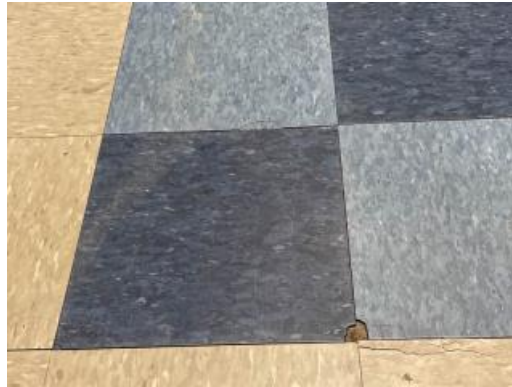
Cracked elevator floor
