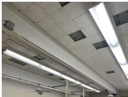
Missing classroom tiles
