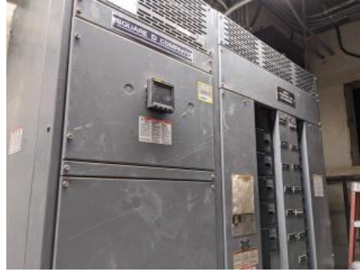
Electrical panel at end of life
