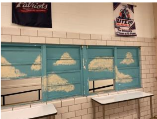
Cafeteria overhead doors at end of life
